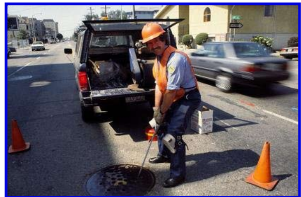
A field services inspector pulls a manhole cover while inspecting for rats.
